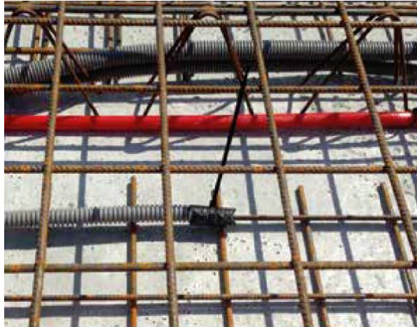
Figure 3.1.8: Sensor installed during the construction phase [2]
